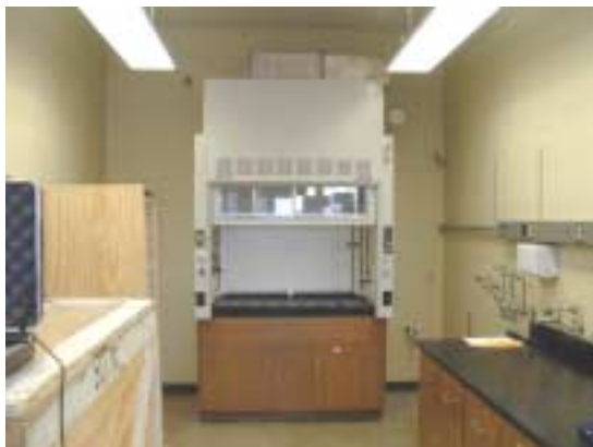
Figure 1 Laboratory Room 214 Fisher Hamilton Test Hood
